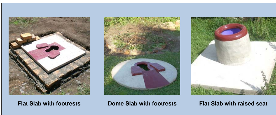
FIGURE 1a. EXAMPLES OF THREE CONSUMER DRIVEN DESIGNS FOR SANITATION PLATFORMS IN UGANDA
